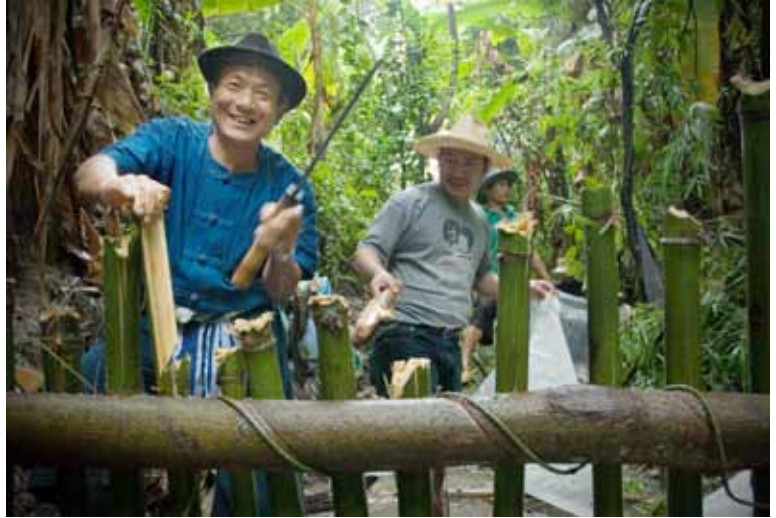
Community members in Nan Province, Northern Thailand, are working together to build a dam that will protect them from more frequent flooding in the area.
